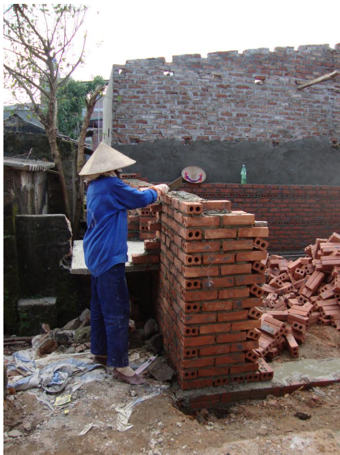
The Cities Alliance project in Vietnam financed studies that led to urban upgrading programs that improved the lives of the urban poor.
