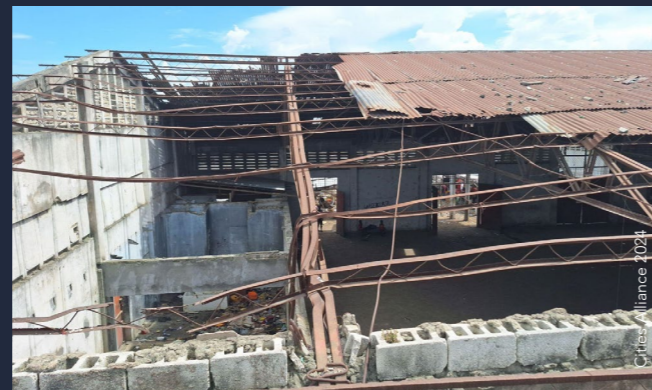
Figure 28 – Structural damage to the roof
