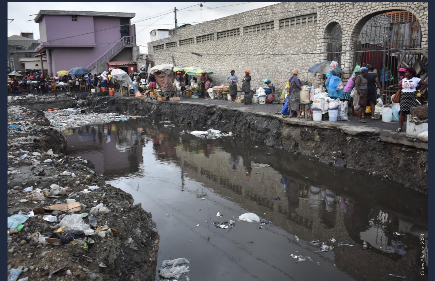
Figure 33 et 34 - Blocked drainage and risk of flooding
