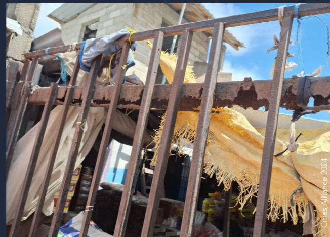
Figure 29 – Damages to commercial infrastructure
