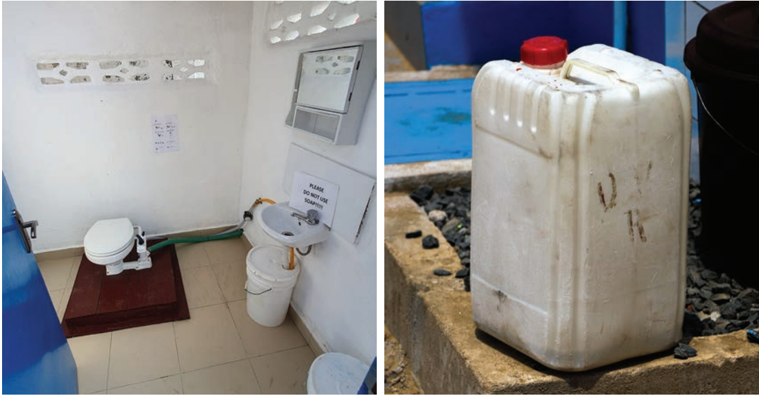
FIGURE 24: Clean Team toilets and services
